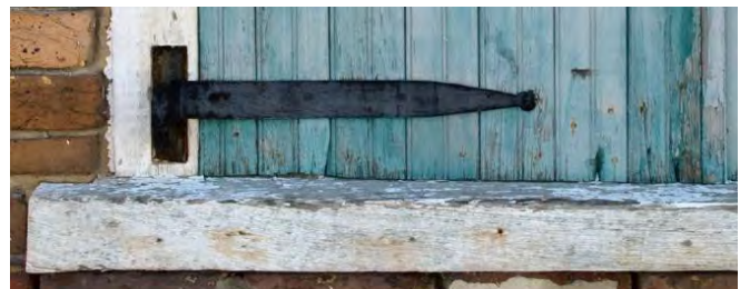
Strap hinges were originally handmade of wrought iron and often painted black. On historic buildings, strap hinges should be simple in design without decorative detailing.
