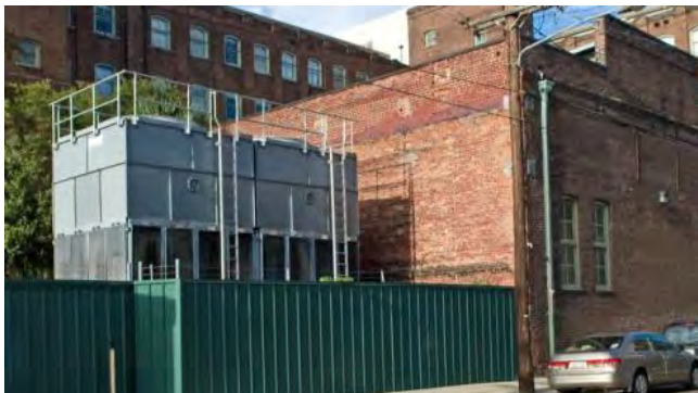
This HVAC equipment is located within this building's courtyard, partially concealed by a fence at a secondary street elevation. It would be preferable if the height of the equipment was lowered to the fence height to minimize visibility.
