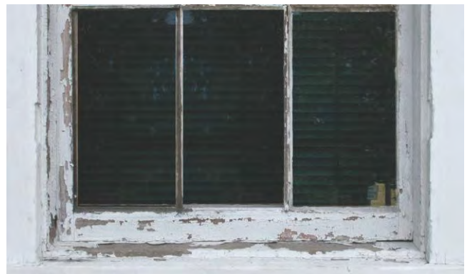
Typically, window deterioration first occurs at the sill. Peeling paint can allow moisture to enter wood and cause rot.
