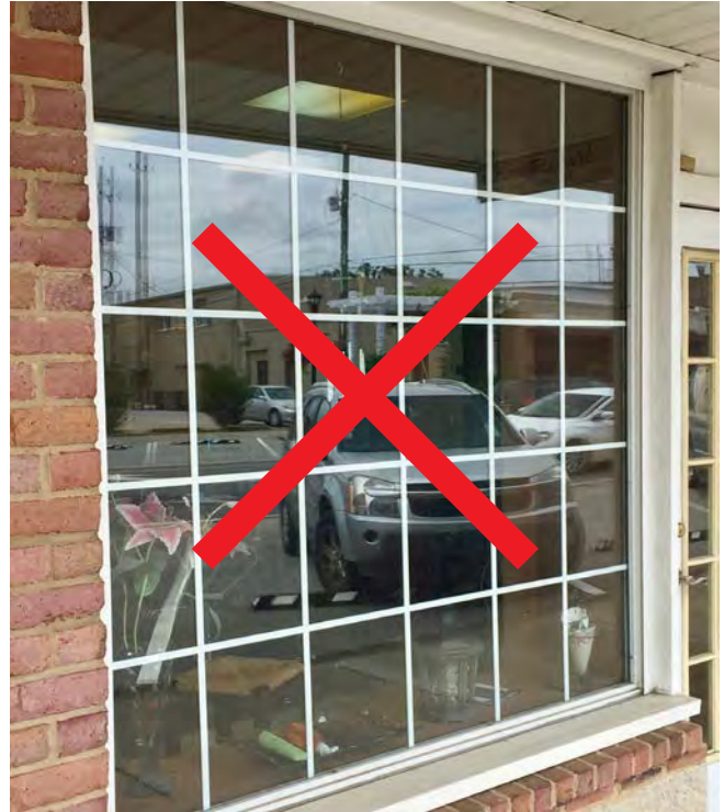
Example of an original storefront window opening that has been incorrectly filled with a vinyl, simulated divided-lite window.
