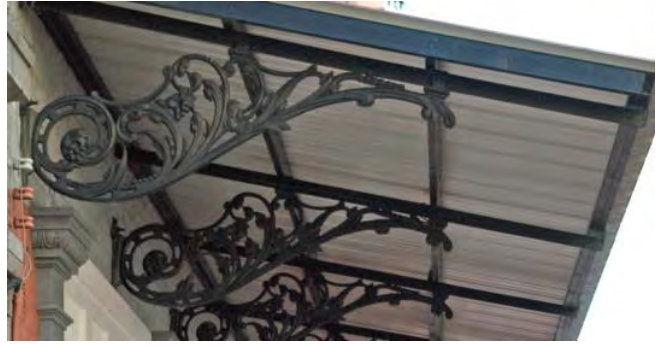
Decorative cast iron brackets and a frame support tongue and groove decking with standing seam roofing above.
