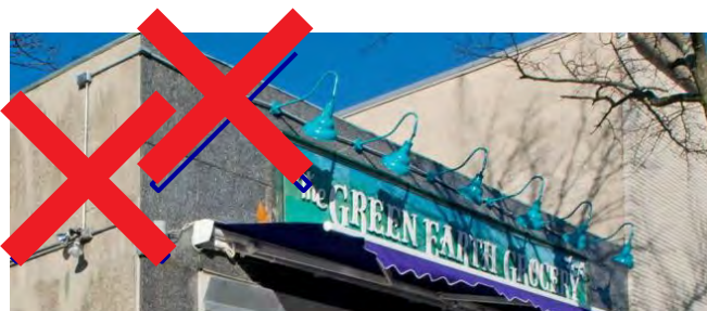
Conduit should be concealed and not mounted to the face of the building. The number of lamps should be reduced to provide enough light for the signs to be read.
