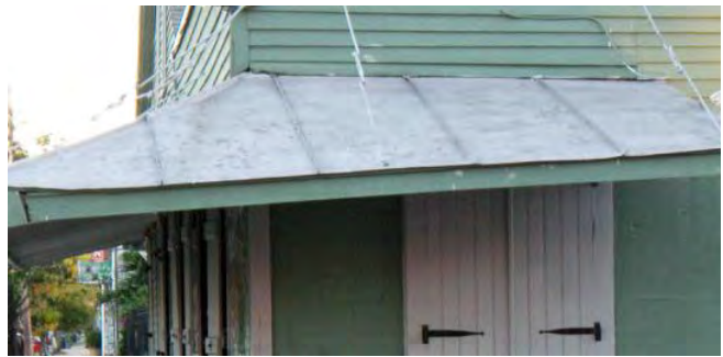
This canopy includes a standing seam metal roof. Canopy supports should be reviewed periodically, particularly where canopies are not level, to ensure they are well supported and not in danger of collapse.
