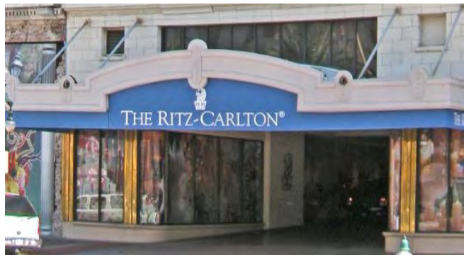
This canopy includes a standing seam metal roof. Canopy supports should be reviewed periodically, particularly where canopies are not level, to ensure they are well supported and not in danger of collapse.
