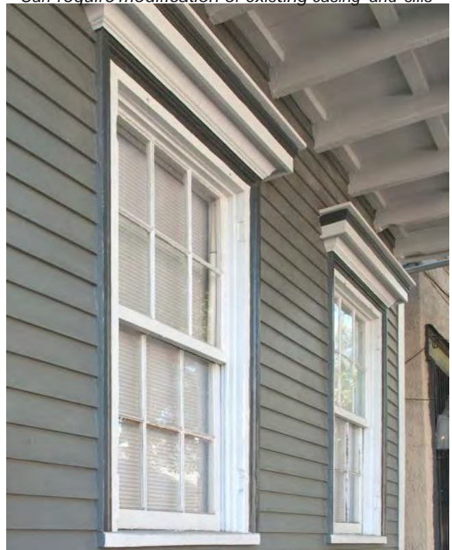
Top Image: The 9/6 vinyl replacement windows in the top image have applied muntins, are mounted flush against the outside wall and lack the depth of traditional windows. They do not have trim or casings including a drip cap and sill. As a result they are inappropriate and would not be approved by the Foley Historical Commission.
