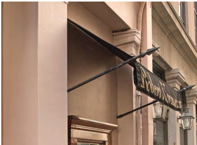
The awning is mounted between the granite piers. The poles are fastened to the stucco surface rather than the masonry, facilitating future repair if removed.
