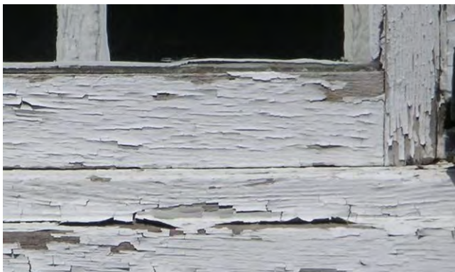
The window sill and jamb have peeling paint and some checking or splitting. Removal of the loose paint will allow the wood to be inspected for signs of rot.
