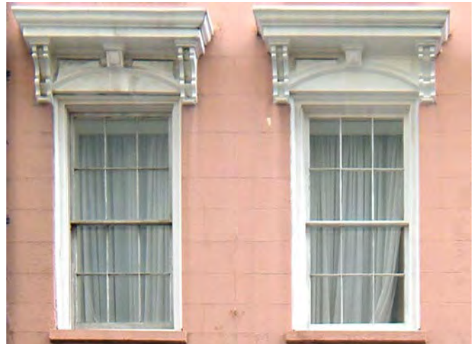
Much of a building's character is defined by its windows. The ornamental cornice above the windows and supporting brackets are typical of the Italianate style.
