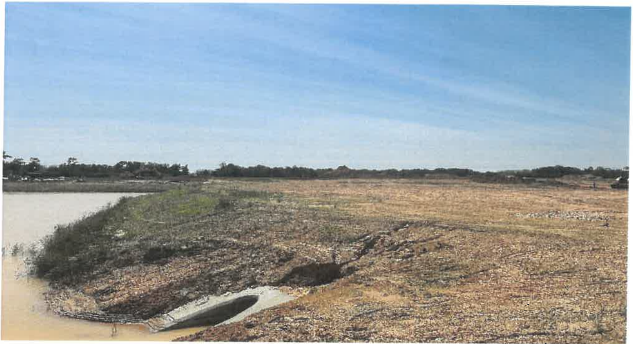
10. Northeast pond Slopes and berm in need of permanent stabilization
