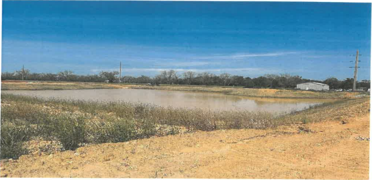
2. Southeast pond inlets & outfall installed. Pond slopes & berm in need of permanent stabilization
