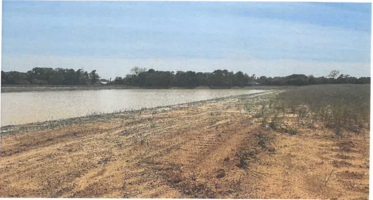
23. Southwest pond in need of permanent stabilization
